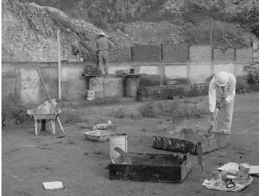
Figure 1 Master Mason Rodolfo Cardenas on the wall and Helper Juan Mata mixing mortar at the Grupo Calider Cal Perla testing location.
