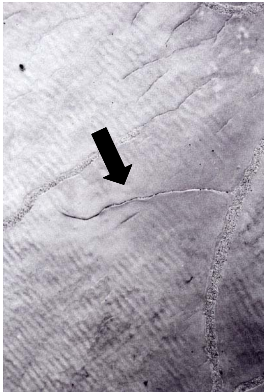
Figure 5: Inspection of DHL filled cracks in 2003 identified failures in exposed locations. DHL had eroded from cracks after a period of one year.
