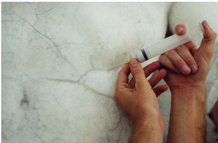
Figure 3: DHL injections beginning in 2001 were intended for filling fine cracks less than 1mm in width. Epoxy injected cracks from the 1996 repair campaign, now yellow in color, are also visible.
