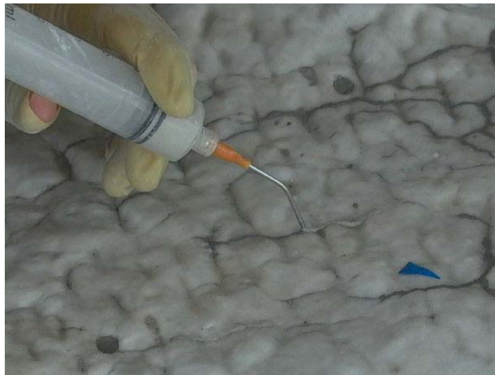
Figure 6: Injection of an NHL cap over a DHL filled crack in 2004. DHL is still wet and appears darker in the crack than the NHL.
