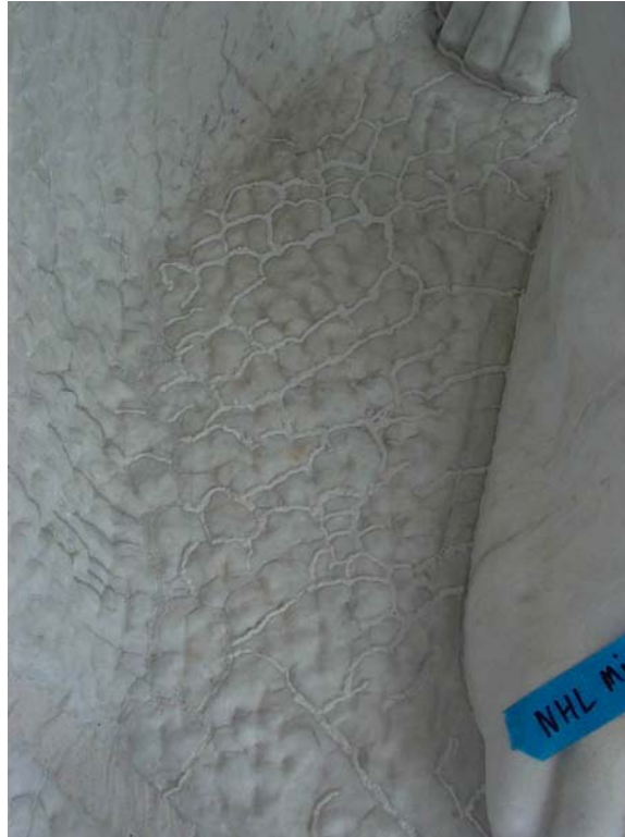
Figure 7: This area of the sculpture base is subjected to water runoff. Here all DHL fills were capped with NHL. This area is not visible from the normal viewpoint of the sculpture and therefore the caps were left proud.
