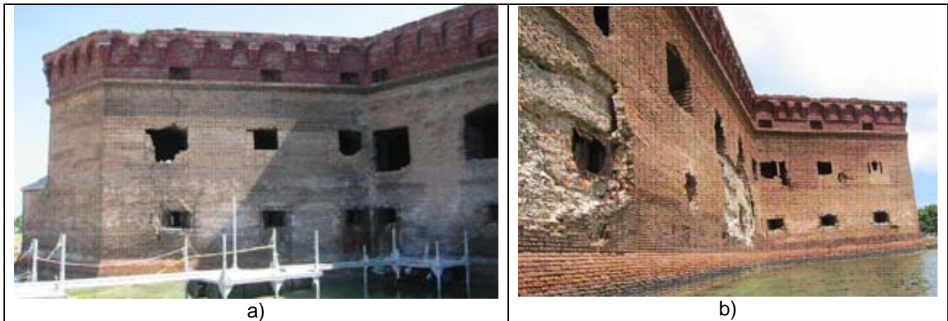
Figure 7 View of Varying Masonry Condition at Fort Jefferson, Dry Tortugas, FL, USA (photograph credit to Martin, 2003)
