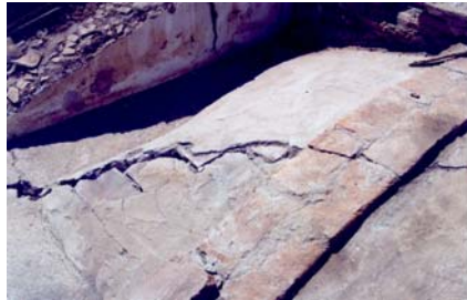
Figure 6- Structural damage on the exterior of the vestry vault
