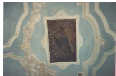
Figure 5- Detail of the lacunae of gypsum plaster at the vault of central aisle
