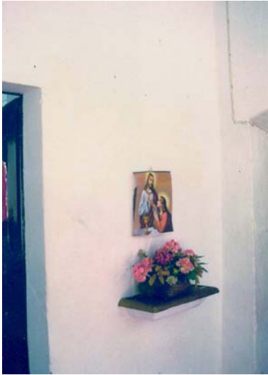
Figure 18- Interior aspect of the sacristy before the restoration
