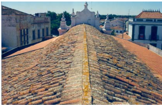
Figure 4- Old roof building. The new tiles seen in this picture belongs to private building adjoining the church.
