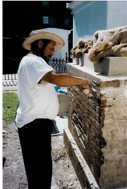
Figure 2. A mason applies a hydraulic lime-based stucco on a step-style tomb. The new material is applied where the original is missing and care is taken to cover the new work with damp burlap (photograph by author).
