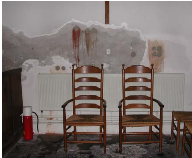
Figure 2 Damage to traditional render as peeling paint layer and finish coat scaling. Caused by cyclical wetting and drying conditions related to rising damp and rain penetration.
