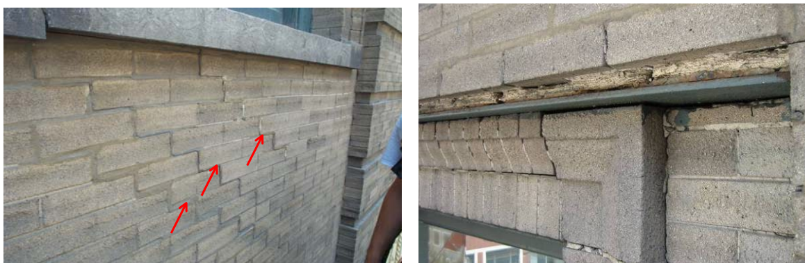
Figures 2 and 3 Representative examples of cracked brickwork at corner (right) and joint conditions (left)
