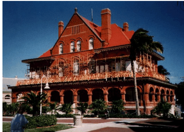
Figure 1. Custom lime-cement repointing mortars for the Key West Customs House simulated, but did not replicate the original mortar, in which poor practices were evident.
