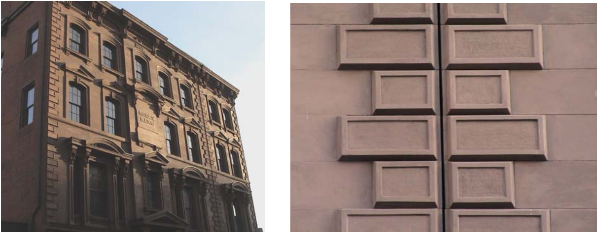
Figure 2. The 1855 Landmark Palladium Building, New Haven, Connecticut (left) shown in 2004, 22 years after application of some 16,000 lbs. of custom latex-modified lime-cement repair mortar. Cast-in-place quoins (right) retain sharp detail, exhibit no evident deterioration and are not readily distinguishable from the original stone.
