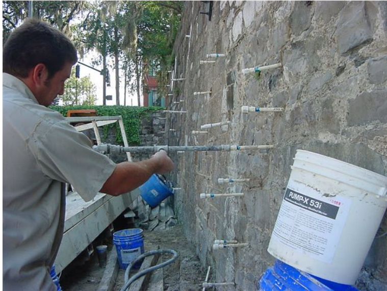
Figure 7. Injection of polymer-modified lime-cement grouts on historic masonry retaining walls on Factors Walk in Savannah, GA, was performed using two different grout formulations.
