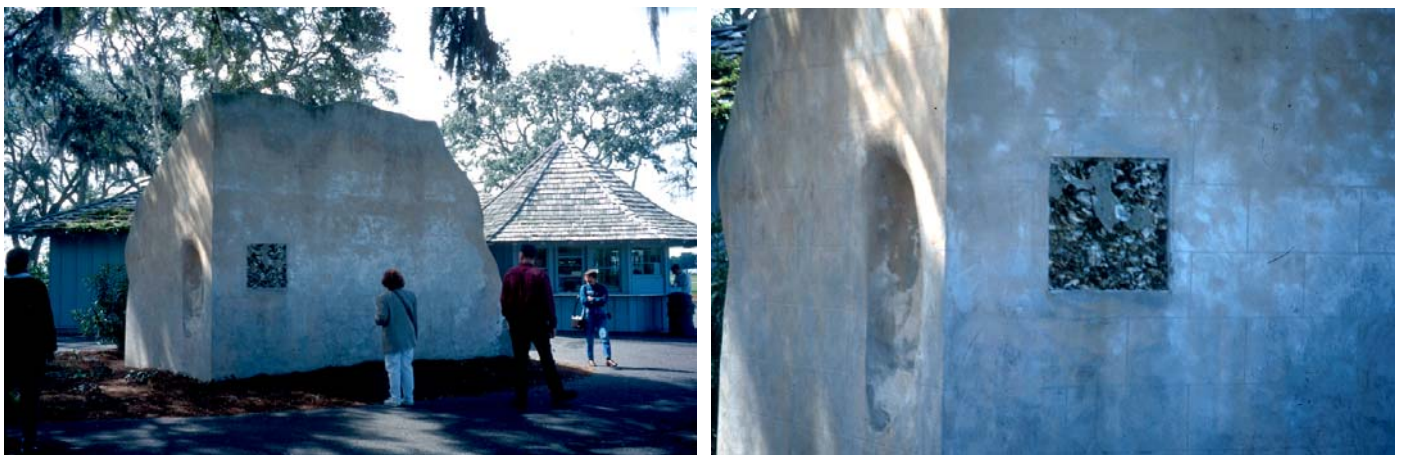
Figure 1 View of the “conserved” remnants of the Retreat Plantation ruins, now within a golf club, on St. Simons island, GA. At right, a detail of the square left without render to show the internal structure of tabby.
